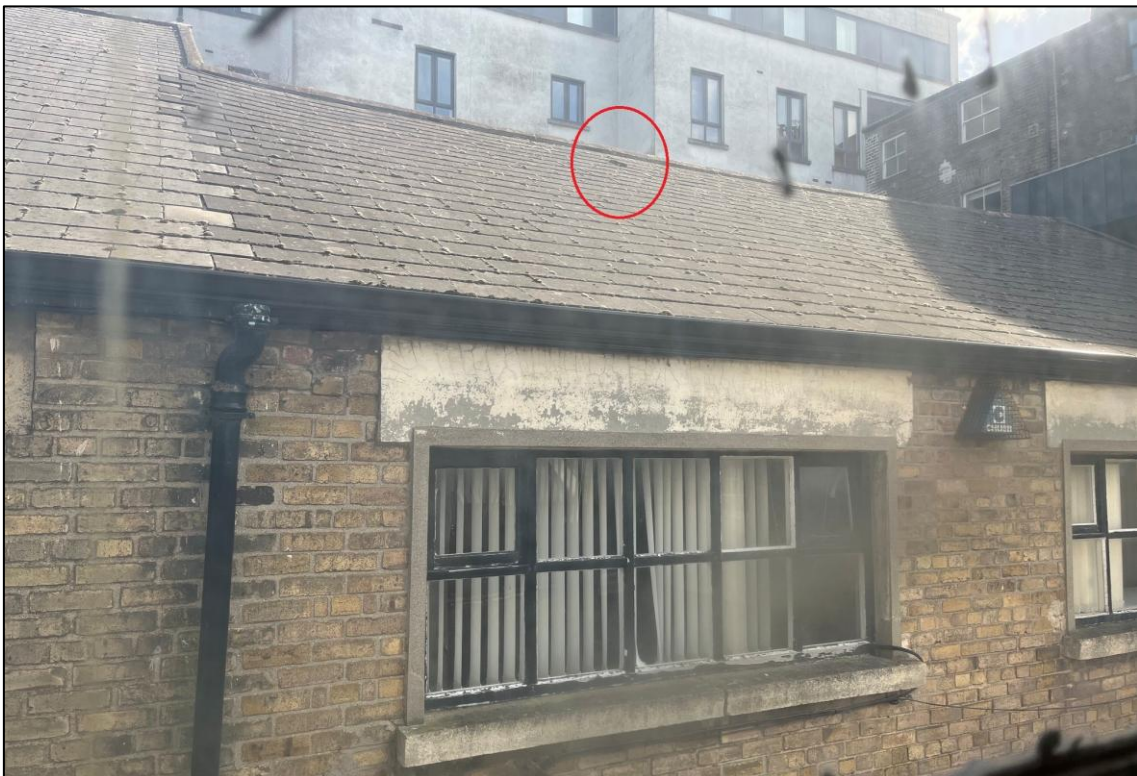
Plate 8: Office building (B2) - Single small gap in lifted tile highlighted in red.
